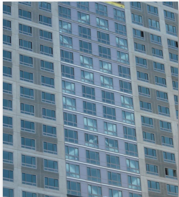
Figure 29: X – braces on 360 State Street
